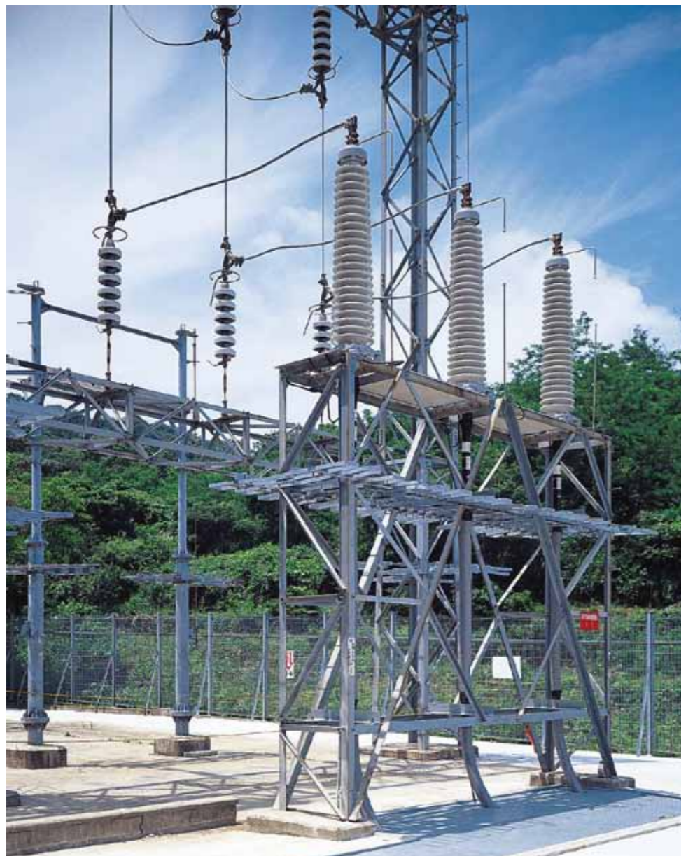
Installed outdoor sealing end
