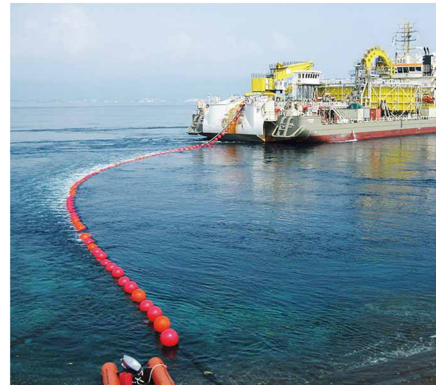
Submarine cable installation under high tidal current by DP-II vessel "Ndurance" in Bali Strait (by courtesy of VBMS)
