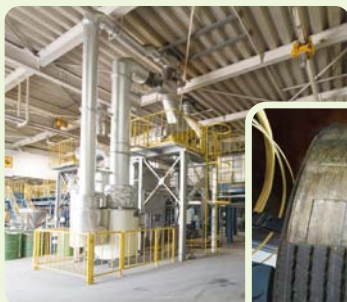
Generation of steam with waste heat recovered from the quenching furnace
