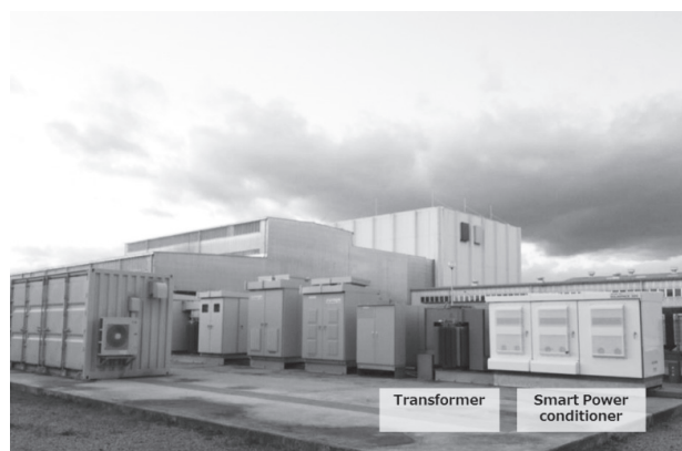
Photo 2. Appearance of field demonstration equipment
